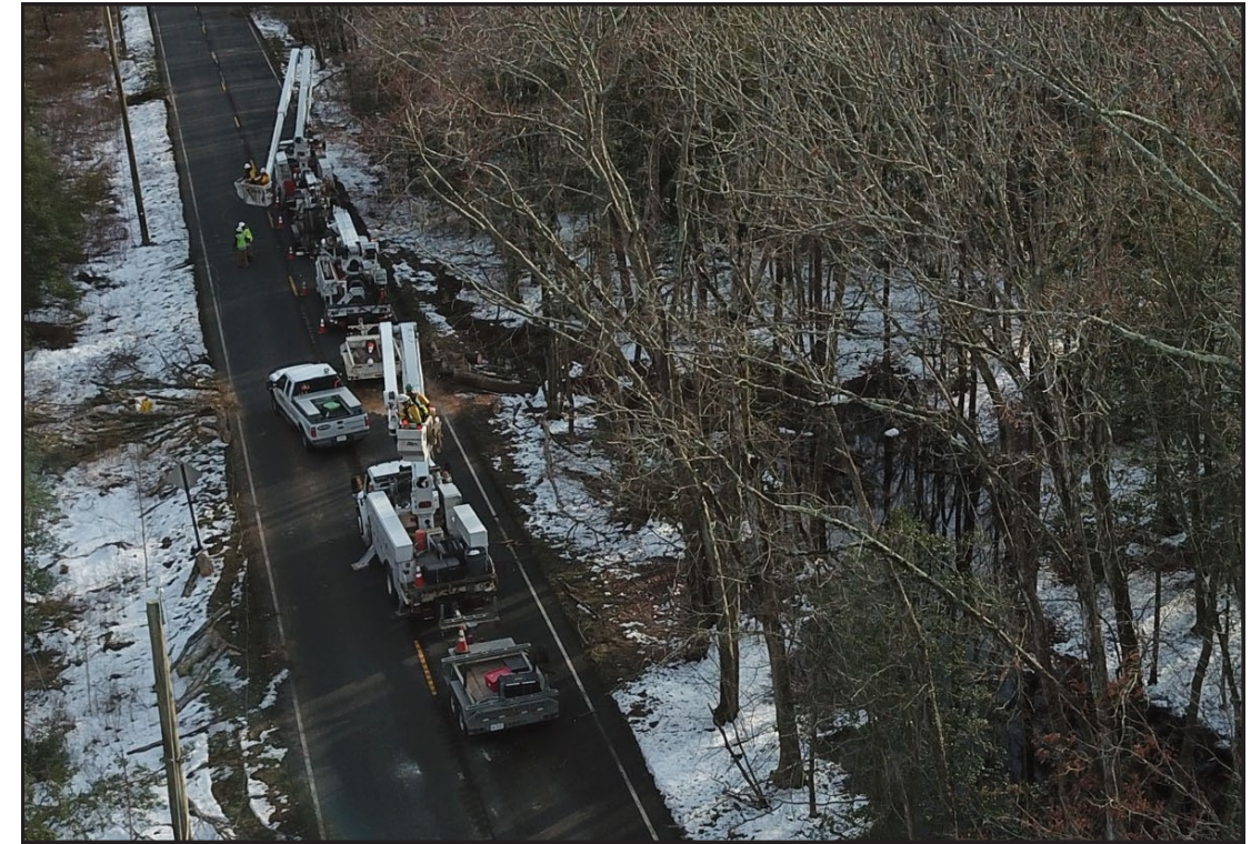
Atlantic City Electric linemen work to repair powerlines and restore power after Winter Storm Toby hit southern New Jersey.
