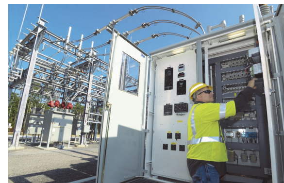
An Atlantic City Electric employee completes work at the company’s new Port Republic substation.
